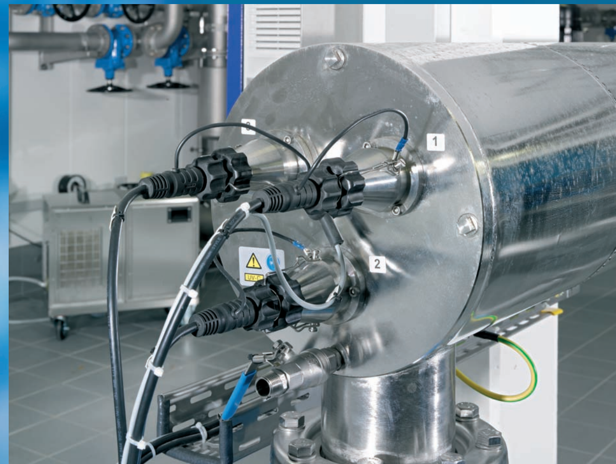
Abb. oben/links: Nanofiltrationsanlage
